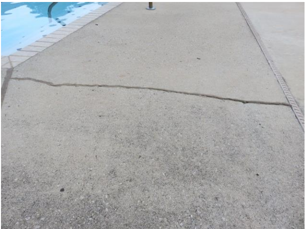
Repaired crack and settlement
