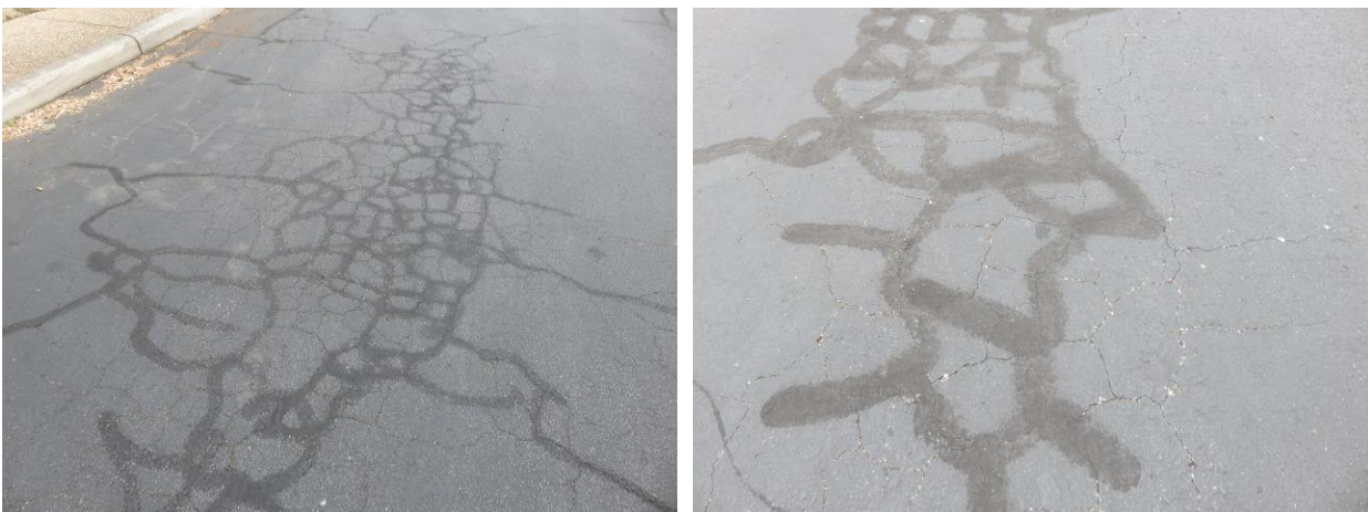
High frequency of cracks
