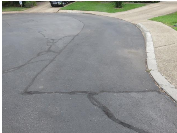
Large patch at cul-de-sac
