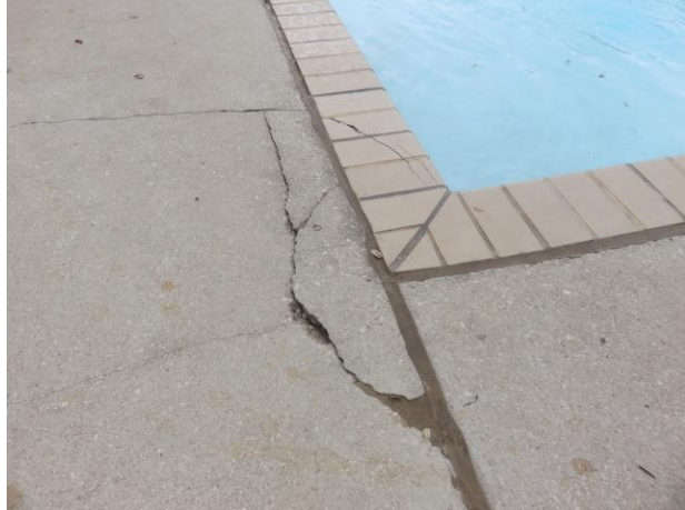
Significant pool deck cracks
