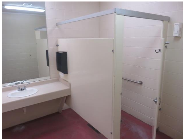
Rest room plumbing fixtures and partitions
