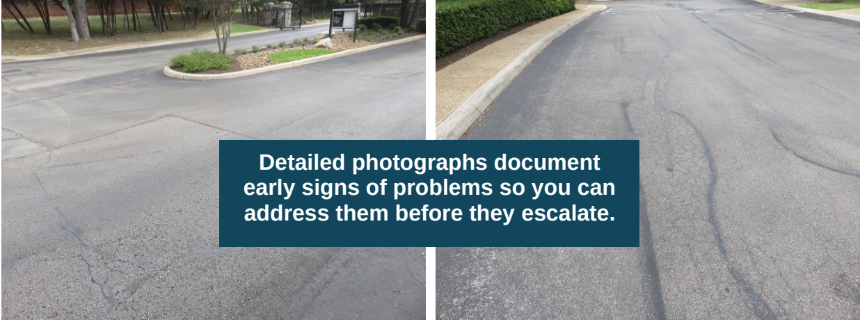
Repaired and unrepaired cracks near gates
