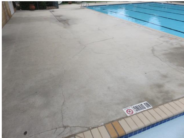
Unrepaired cracks throughout section of pool deck
