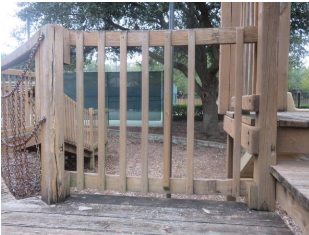
Missing spindle at playset railing
